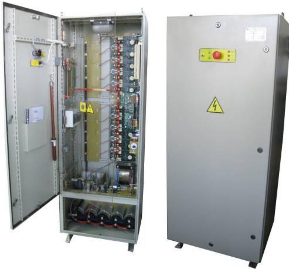
Fig.7 Power block of installation IM3
