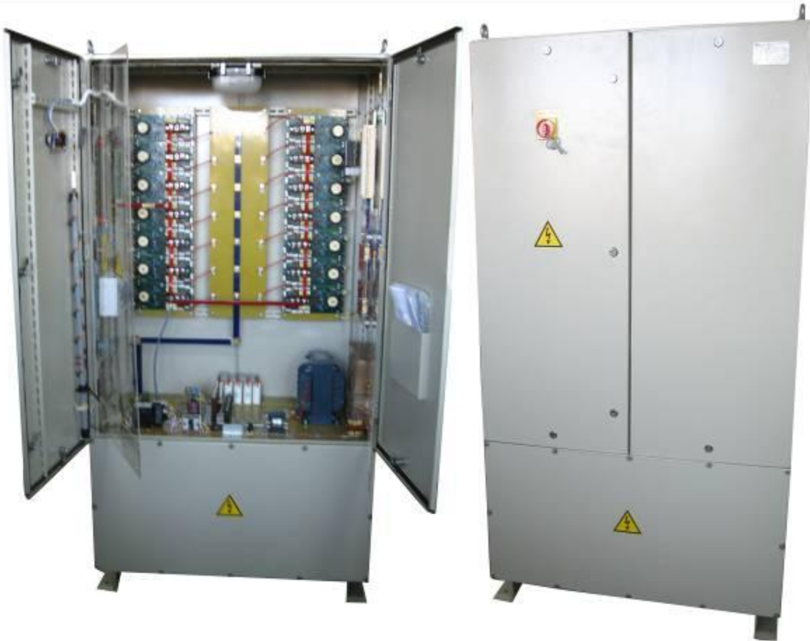
Fig. 8 Power block of installations IM4, IM.
